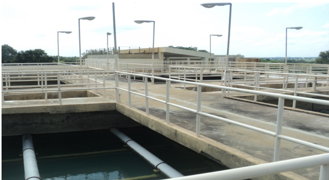
Fig. 1. ABU water treatment plant.
