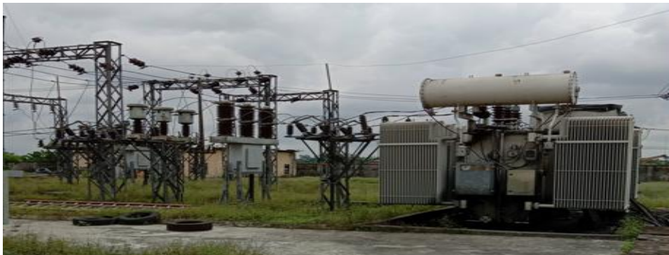
Fig.2. Otovwodo 15 MVA injection transformer and switch yard.
