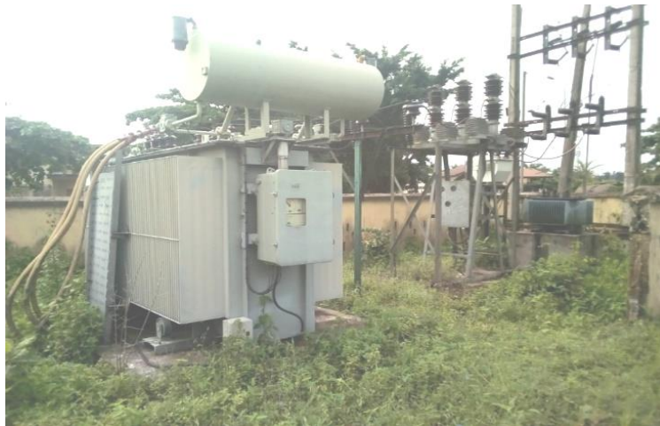
Fig. 3. Photo view of DELSUTH 7.5MVA, 33/11 Transformer Substation.
