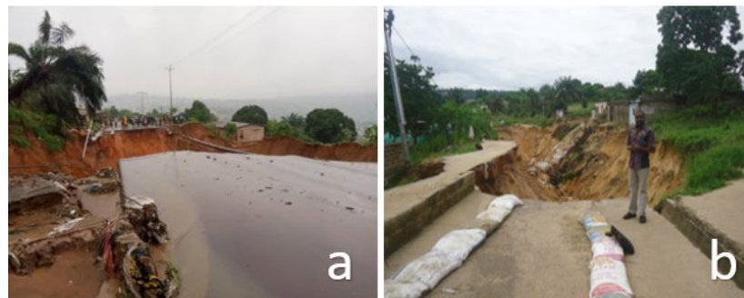
Fig. 3. Images with the affected road infrastructure: a) National road no 1 cut by a ravine; b) University of Kinshasa-Kimwenza road cut by the ravine.
